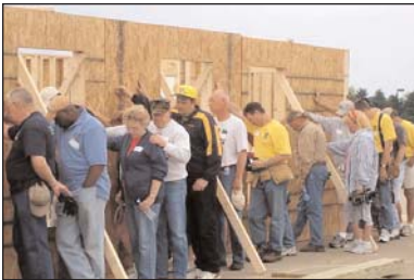
Christians from a variety of churches in Lexington pray over the home they built for New Orleans.
